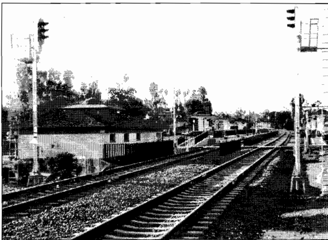
The Sprinter station at Vista nears completion, but signals facing each other still have a way to go. Photo by John Ulloth
