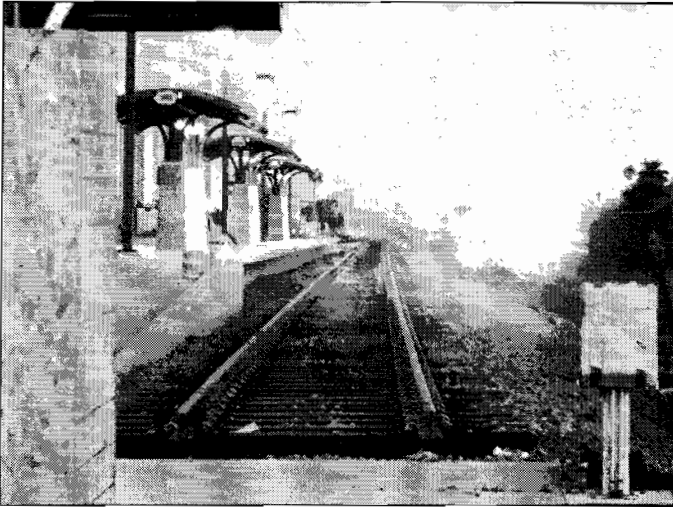
Western track of Sprinter's Oceanside Terminal is still under construction. A northbound Amtrak Pacific Surfliner passes on the right. Photo by John Ulloth
