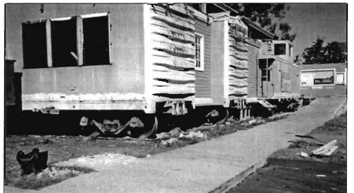
Demolition of the Sea Food Grotto in Torrance – exposing three rail cars (2 box and 1 caboose) which formerly were part of the local Victoria Station Restaurant, somewhat similar to the original in Universal City. Note they retained their running gear on track. Photo by Jack Whitmeyer
