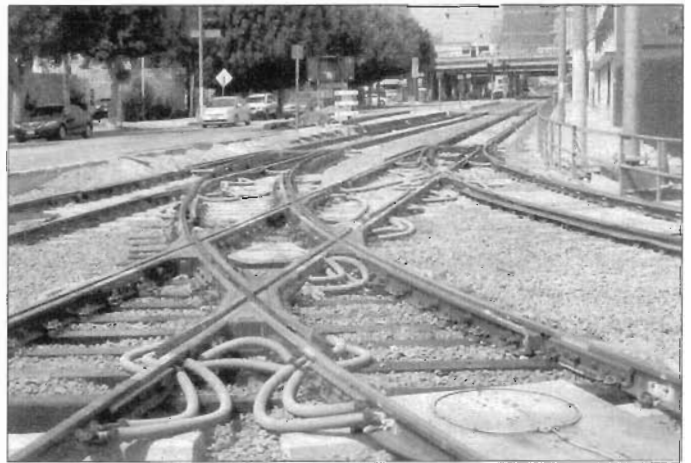
Expo Line connection with Blue Line at Washington/Flower (view north) in May 2010. Note concrete ties for turnouts and wood ties for crossing diamond. Photo by John Whitmeyer
