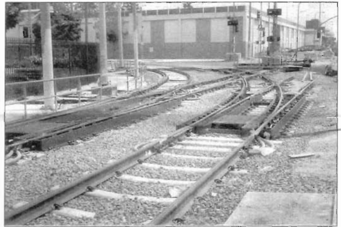
Exposition Line junction connection with Blue Line at Washington Blvd./Flower St. (view south). Photo by John Whitmeyer
