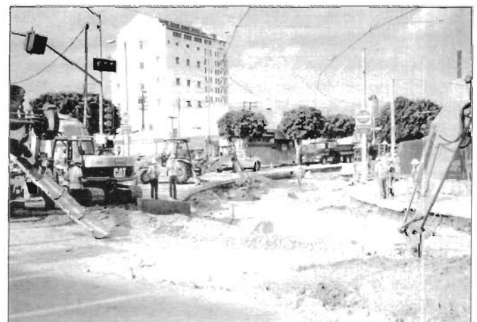
Track renewal of Metro Blue Line is seen at Washington/Flower Street curve in Los Angeles. Photo by John Whitmeyer
