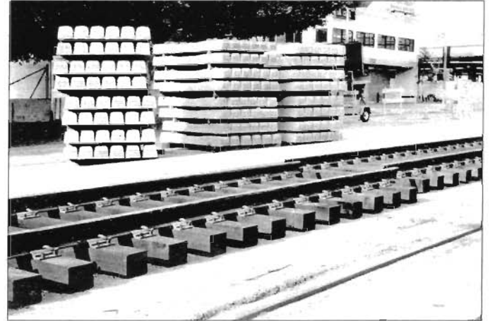
Seen on Nov. 21 are concrete ties and temporary track panels for Metro Blue Line track renewal. Photo by John Whitmeyer
