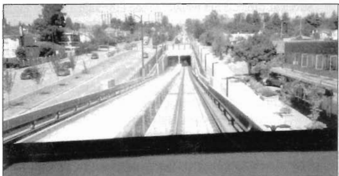
View is north at point where the "Canada Line" goes underground in cut-and-cover along Cambie Street in Vancouver, British Columbia. Photo by John L. Whitmeyer
