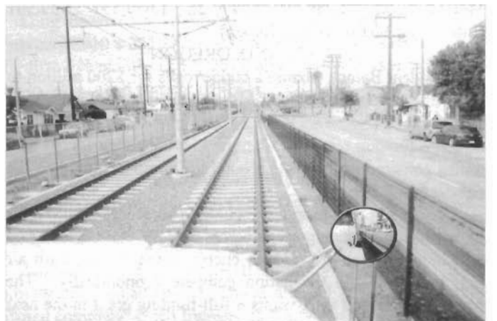
Testing of track geometry of Expo Light Rail Line during construction — looking west. Image by Metro
