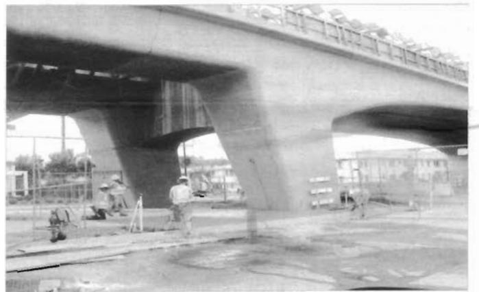
Concrete placement of East Pedestrian Plaza at La Brea Aerial Station during construction. Image by Metro
