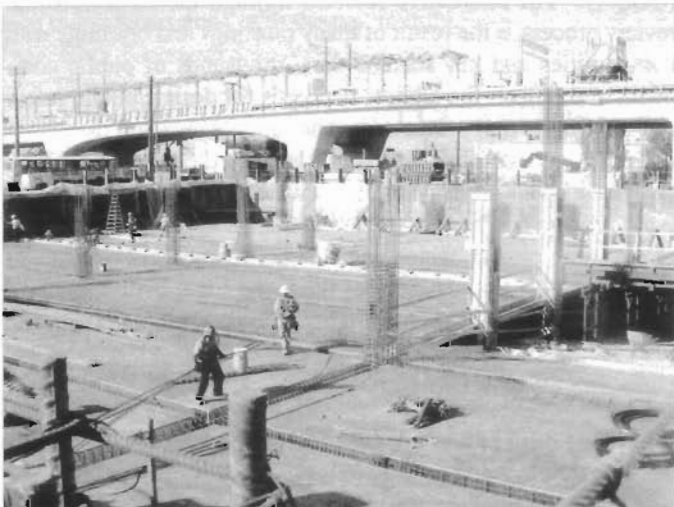
Rebar installation at La Cienega parking structure of Expo Light Rail Line during construction. Image by Metro
