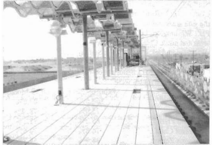
La Cienega Aerial Station platform during construction — looking west. Image by Metro
